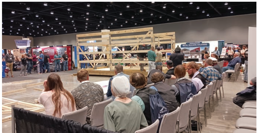
Attendees could watch a small building put up in real time, right on the expo floor, by a crew unfamiliar with the Rapid Framing System. PHOTOS BY SHIELD WALL MEDIA
