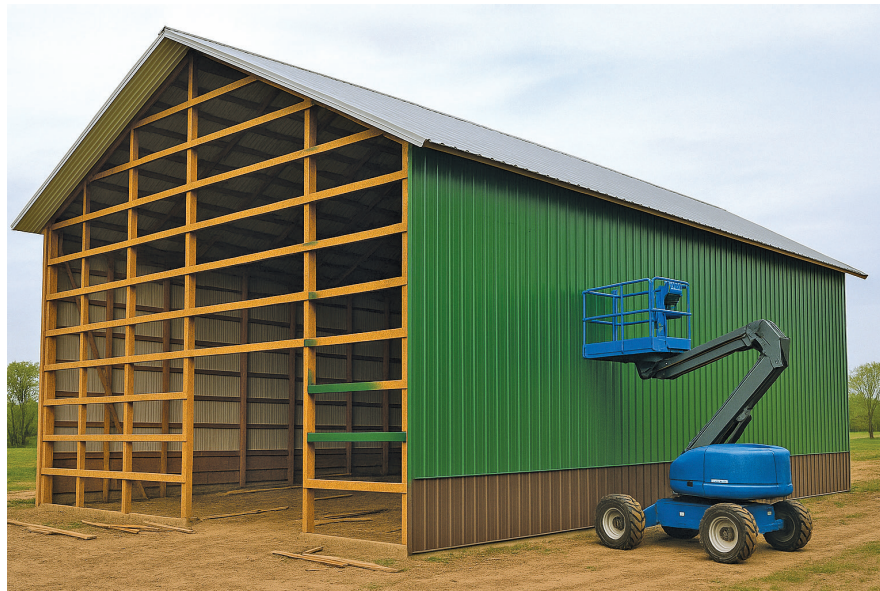
When the building perimeter is clear, it helps prevent delays and ensures a clean, safe workspace throughout the project.
