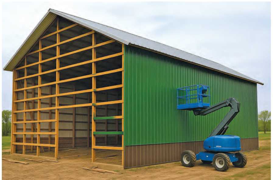
When the building perimeter is clear, it helps prevent delays and ensures a clean, safe workspace throughout the project.
