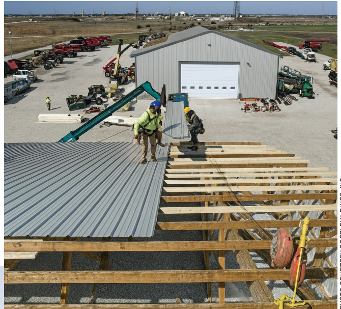
Steel is the most popular choice for reskinning an existing post-frame building.
