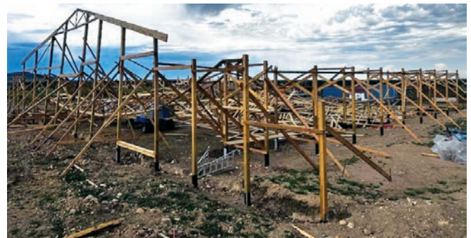
Significant damage caused by high winds.
