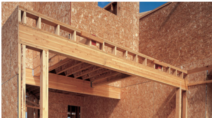
The ability of glulam beams to span long distances and their dimensional stability makes them an ideal option for garage door headers. (PHOTO BY THE APA)
