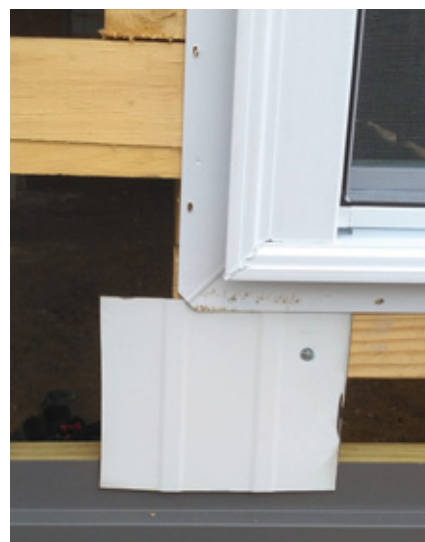
Builder Roger Higginbotham places a small piece or strip of scrap steel under window corners.
