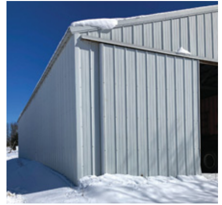
Snow around a building can lead to water intrusion.
