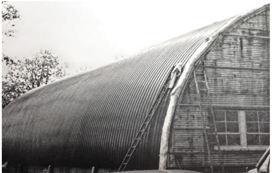
A 4 high mechanically attached ribbing not only provided the anchor for the metal sheathing, but provided ample room for badly needed insulation.
